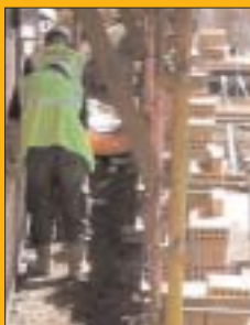
Figure 2 Brick stacks are placed on the system scaffolding to raise their height and reduce the amount of bending required. The wide trench next to the scaffolding enables materials to be delivered onto the scaffold
