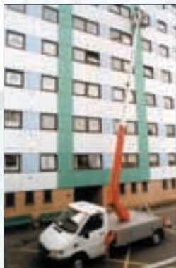
DL21T at inspection by a block. The 5th or 6st floor is reached easily and safely.
